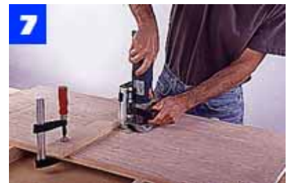
Cut the plate slots in case parts. Clamp a straightedge to each upper case shelf to position slots for center partition.
